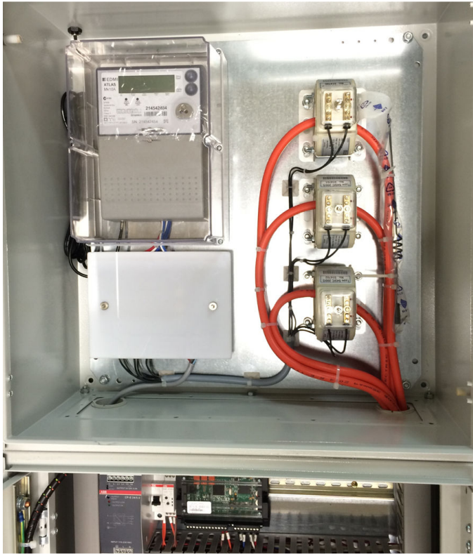
Export Allowed with Utility Consumption meter
